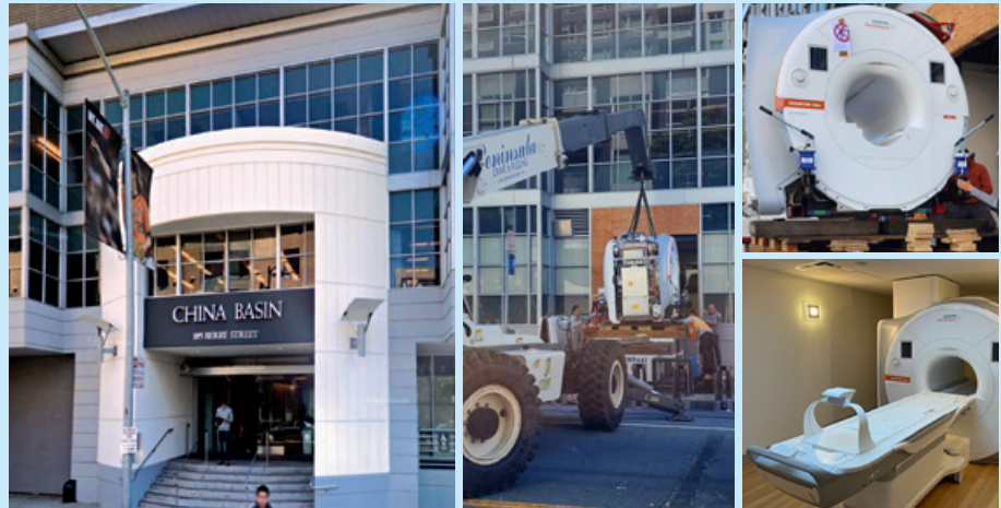
Delivery of the Siemens MAGNETOM Sola 1.5T MRI to the China Basin Landing site in San Francisco. (Installation photos by Alastair Martin and Craig DeVincent.)
